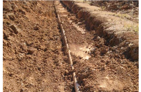
Bonded asbestos pipe uncovered in soil
